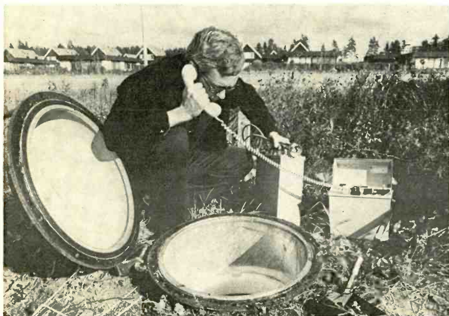
SIEMENS ENGINEER CHECKS an underground repeater on 60-MHz Örebro-Västerås line.
